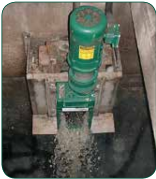
Muffin Monster grinder in a pump station
