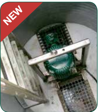
Muffin Monster Manhole at a correctional facility
