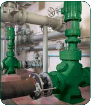
Muffin Monster in-line grinders in a pump station
