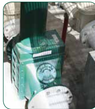
Macho Monster in-line sewage grinder in a jail
